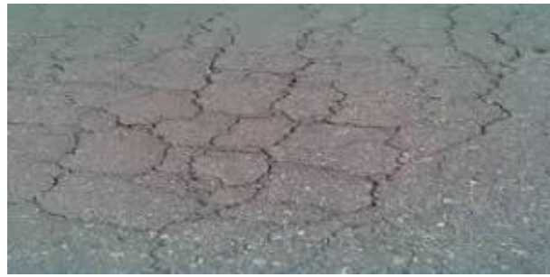
Figure 10. Block Crack Damage
