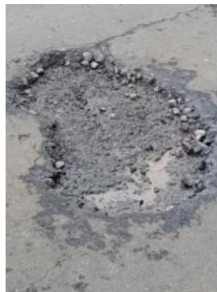
Figure 9. Grain Release Damage
