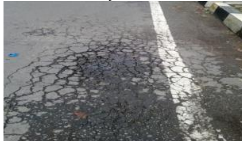
Figure 8. Crocodile Skin Cracks
